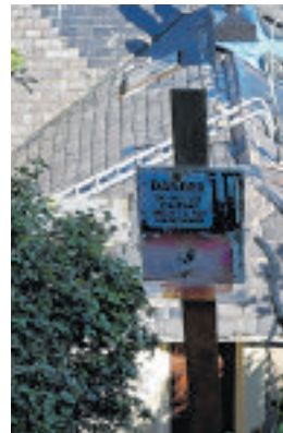
Danger sign and roof repairs
