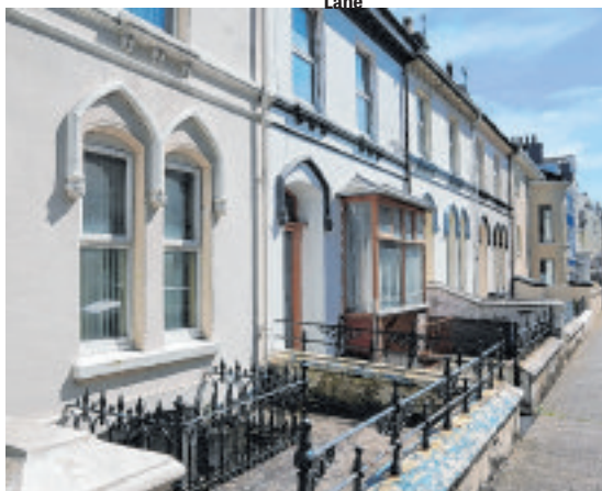
A change to the ground floor windows of one property in a terrace
