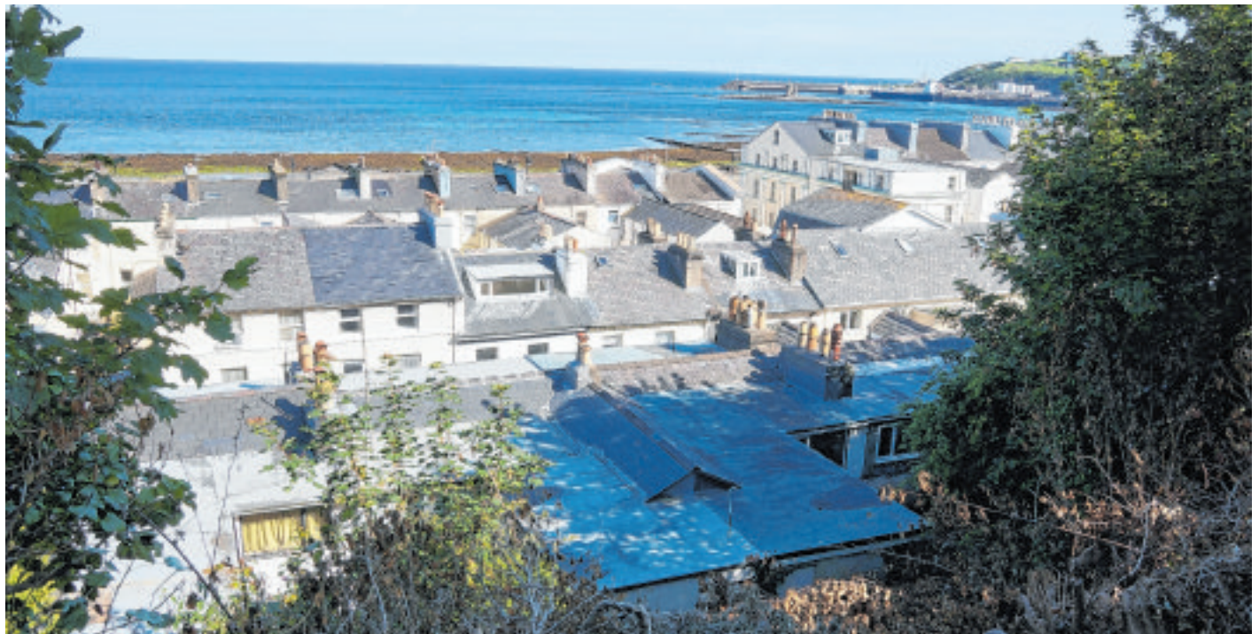
Alterations to roofs and rear outlets of Castle Mona Avenue and the reopened view
