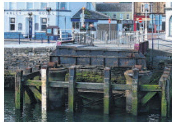
The iron piles which support the ends of the bridges when it is in use
