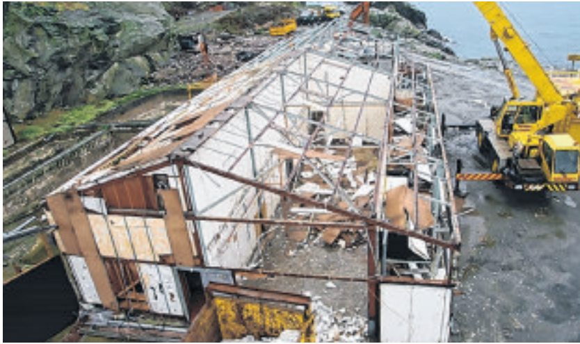
Demolition of the 1963 'white fish' extension in 2006, with spawning ponds visible between the building and cliffs (photo: Culture Vannin)
