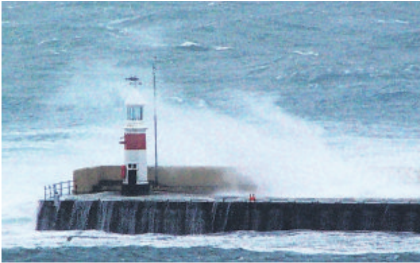
Port St Mary's light under bombardment just before it was washed away
